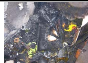
December 14, 2006 Structure Fire
